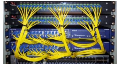
Optical Central Unit (OCU) installed in server room
